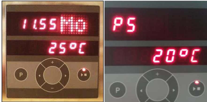
Fig.: Start on control panel
