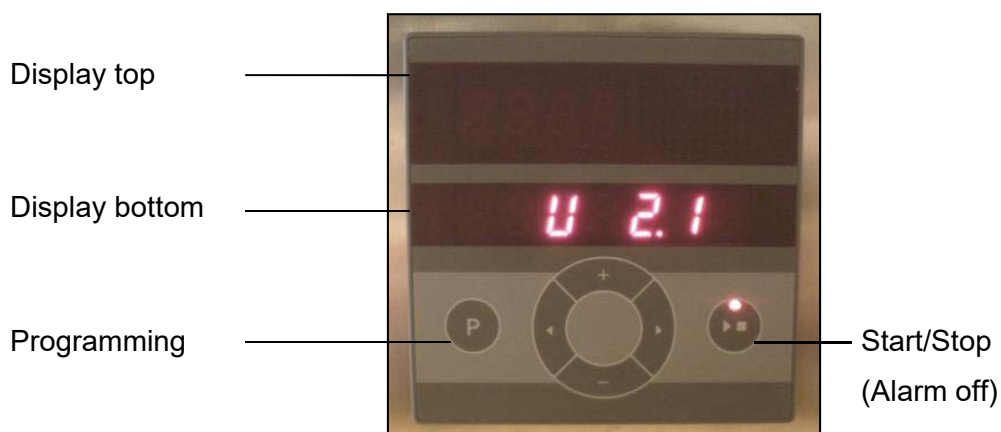
Fig.: control panel
